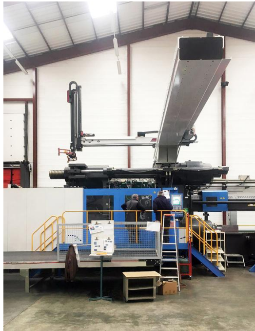
WITTMANN WX193 robot – the first of its kind – during installation work in April 2019.
